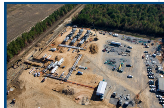
Chesapeake: North Louisiana Natural Gas Treating Facility.
